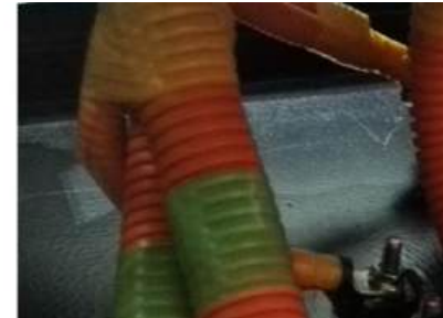
The ground wiring harness are fixed and intact
