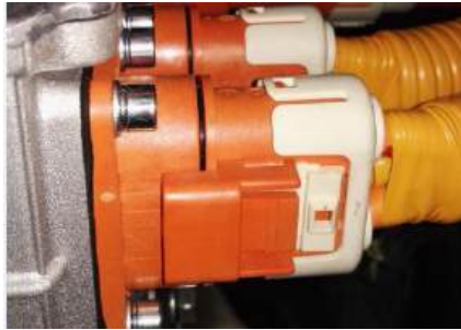
High voltage connector of charging port is in normal state
