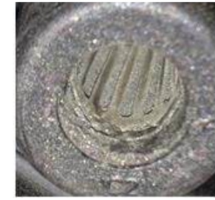
Terminal broken and falling off
