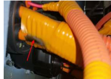
Blackened outer layer of cable at tail end of the charging port
