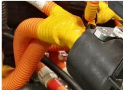
Normal cable at tail end of the charging port
